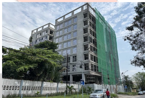
Av. Justice Building Kinshasa – Dr Congo Fire Detection, Fire Fighting and Plumbing
